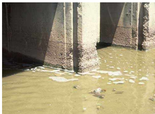
Figure 1.3: Characteristic degradation of a concrete bridge pylon in the Pimpama River, southeast Queensland [7]
